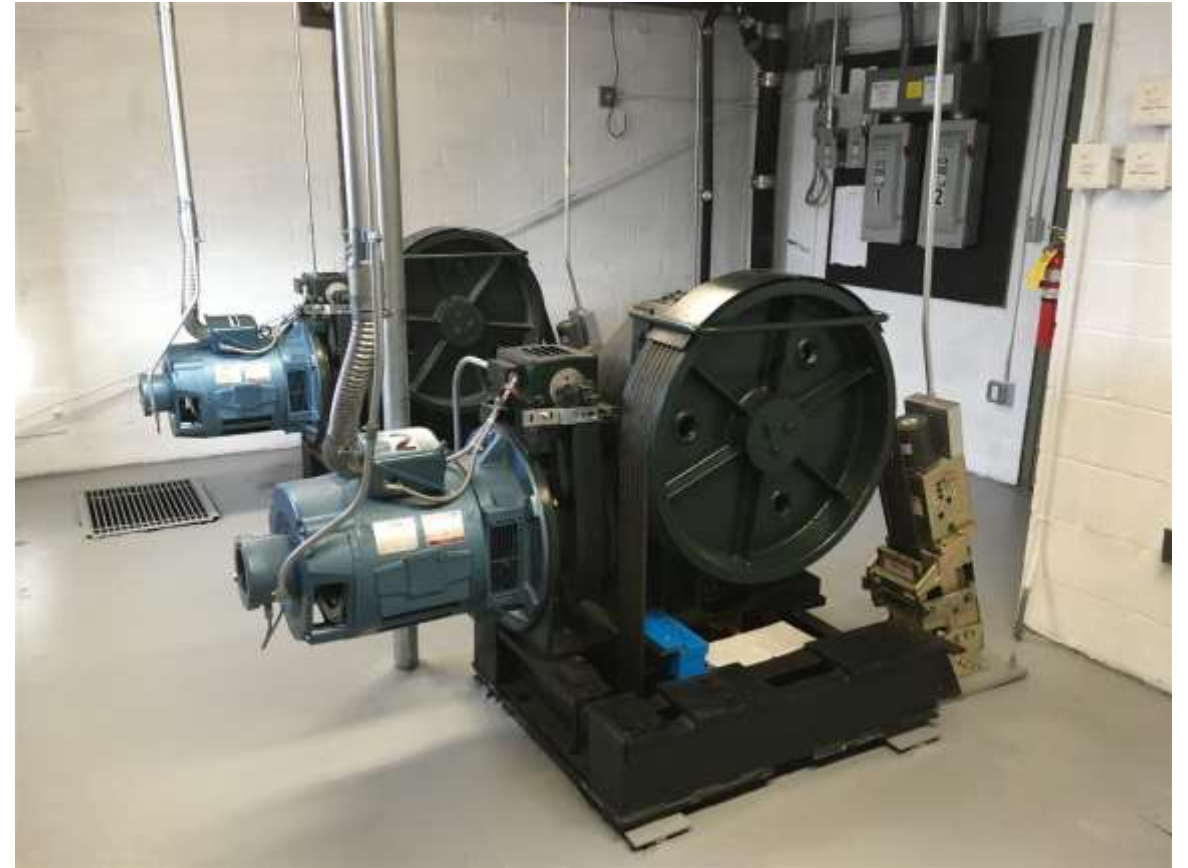
New AC Motors, Cable Brake
