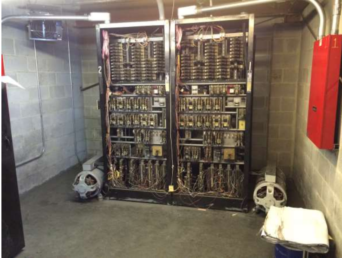
Old Electronics and AC to DC Generators
