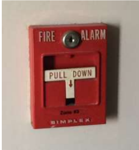
Old Alarm Pull
