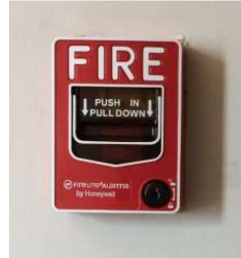
New Alarm Pull
